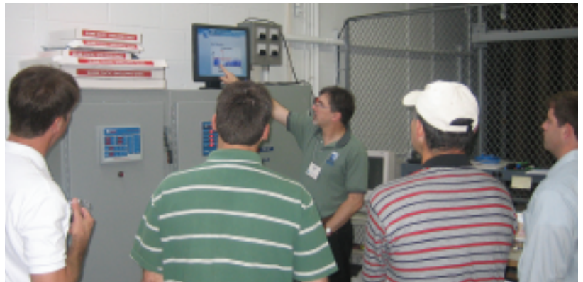
Bela Toth explains MVC operations in a drill session. From Left to Right: Steve Martin (E.I. DuPont, Pass Christian, MS), Chuck Ashworth (Associated Electric Cooperative, Inc., Clifton Hill, MO), Bela Toth (Neundorfer), Greg Woods (Associated Electric Cooperative, Inc., Clifton Hill, MO), Jim Silk (AEP, Columbus, OH)
